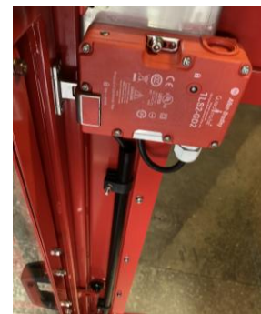
Safety Door Locking System
